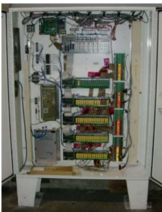
Old Control Panel
