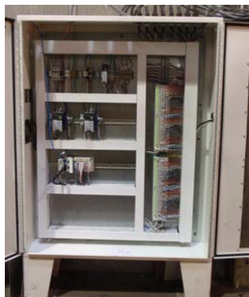
Upgraded Control Panel
